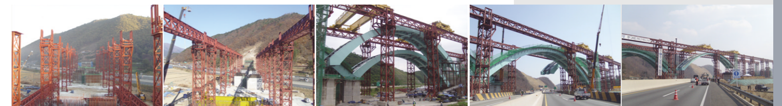
① Install Temporary Supports ② Install Temporary Truss ③ Assembling Steel Arch ④ Lifting Steel Arch ⑤ Install Steel Arch
